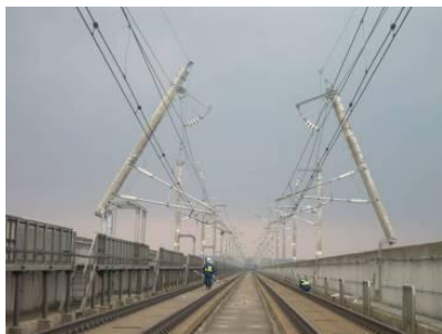
Broken, leaning, or cracked electrification masts
