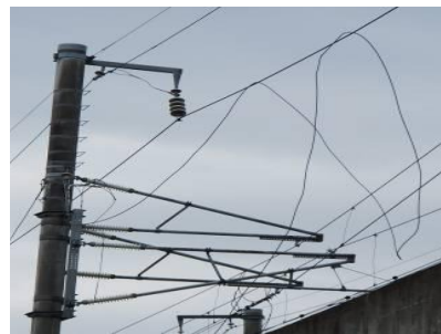
Severed power lines
